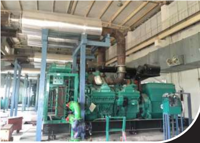
DG Sets, Honda Car Plant - Rajasthan
