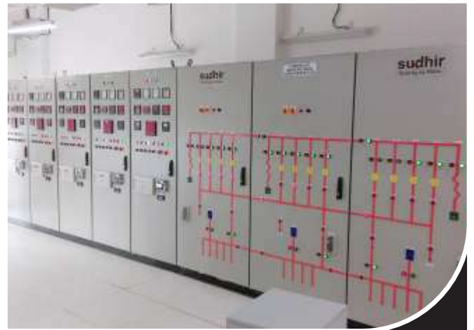
Panels, Reliance IDC - Maharashtra
