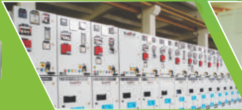
Sudhir - Schneider HT Panels
