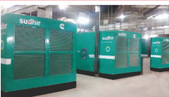
Sudhir powering 1600 bed multi-speciality Safdarjung hospital , New Delhi
