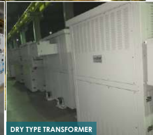
DRY TYPE TRANSFORMER
