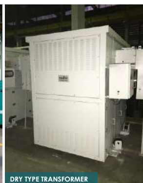
DRY TYPE TRANSFORMER
