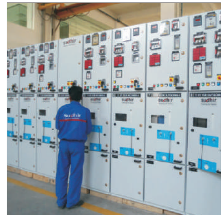
33 kV HT Panel
